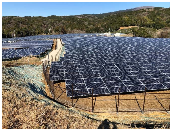
Power plant whole view
